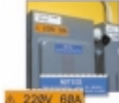
Electrical Panel Identification
